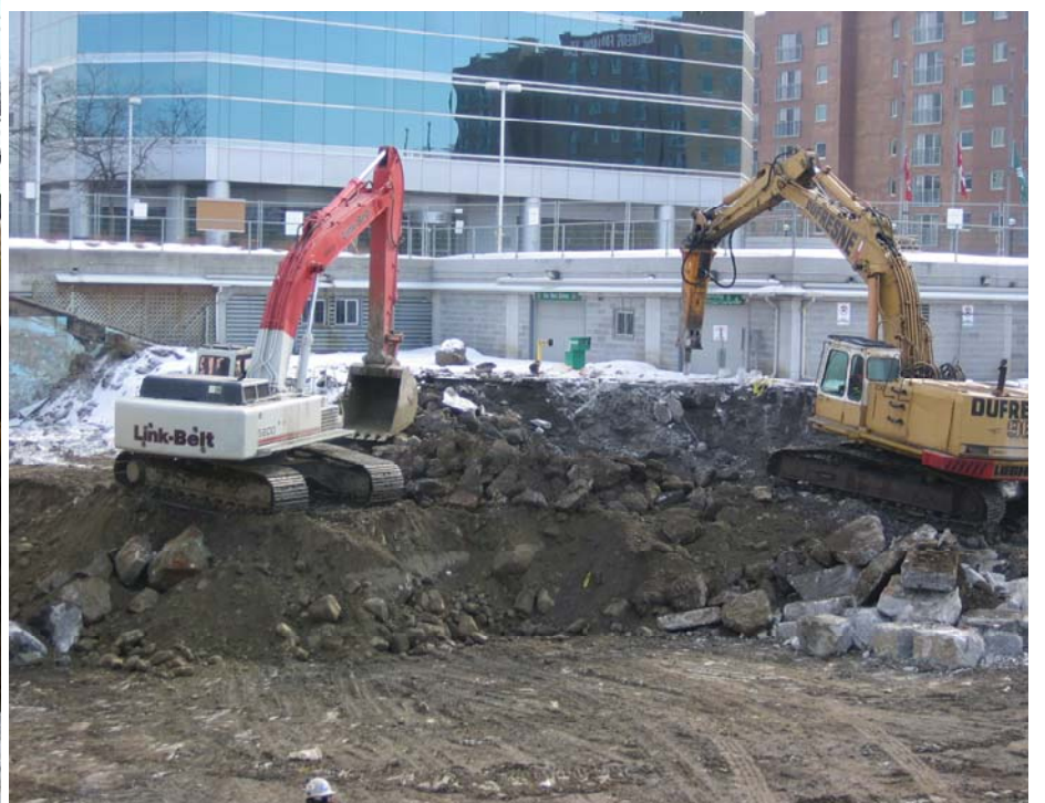
Impacted soil at a commercial facility, Ottawa, Ontario
