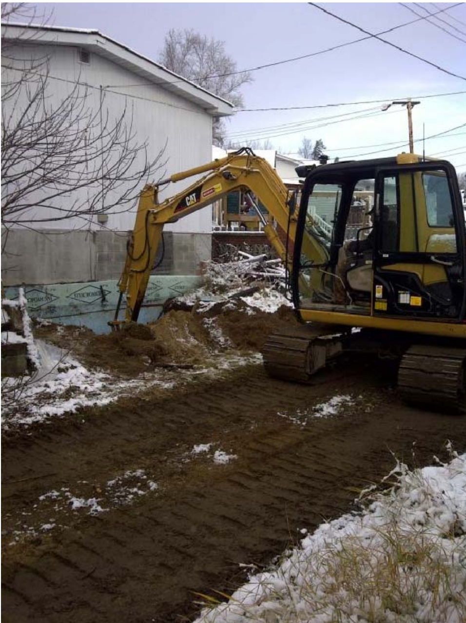
Impacted soil at a residential property, Timmins, Ontario
